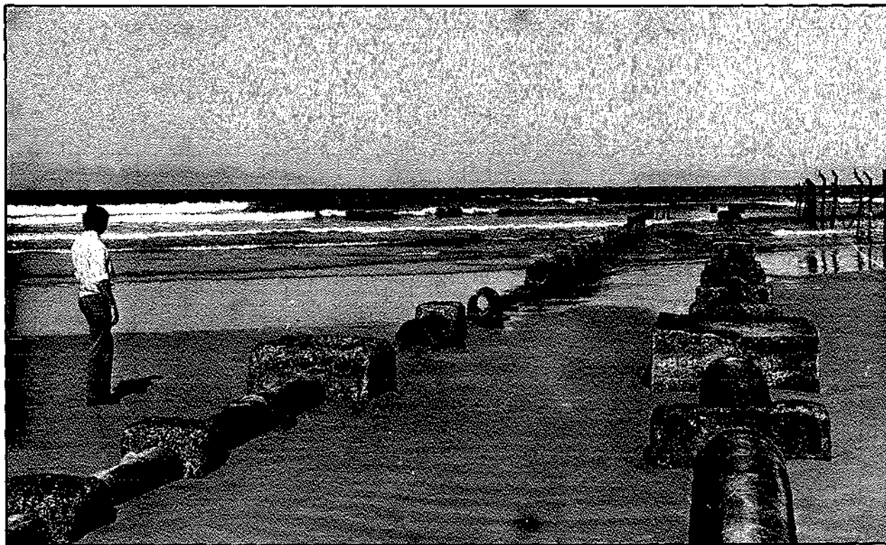
A discharge pipe which transports effluent from a fruit processing factory to the sea
